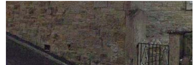
Figure 28: Rubble Stone to all elevations fronting the street. Use of quoins only on key junctions (cross roads). Random coursing.
