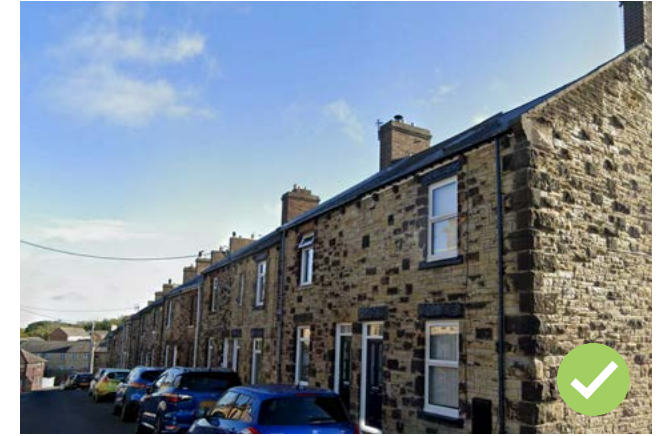
Figure 23: Positive use of traditional rubble stone in terraced facades, which is locally distinctive and creates interesting texture. Uniformity of architectural materials and elements along the street.
